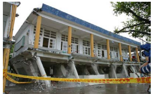
In-situ pushover test to verify the proposed technology for seismic evaluation and retrofit of school buildings
