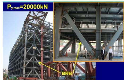
The Buckling Restrained Brace applied to Taichung City Government Building
