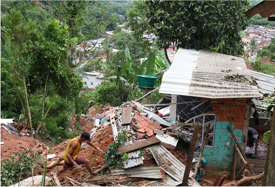
Figure 8 – Very simple houses destroyed by landslide in Vila do Sahy village, São Sebastião municipality in February 2023 (Source: Rovena Rosa/Agência Brasil)
