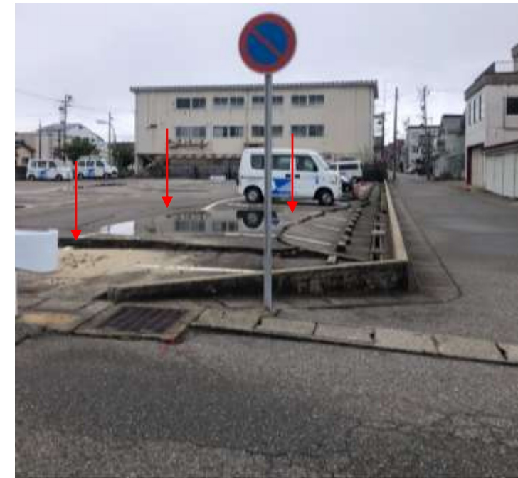
Cracks and ground subsidence at parking lot near bridge
