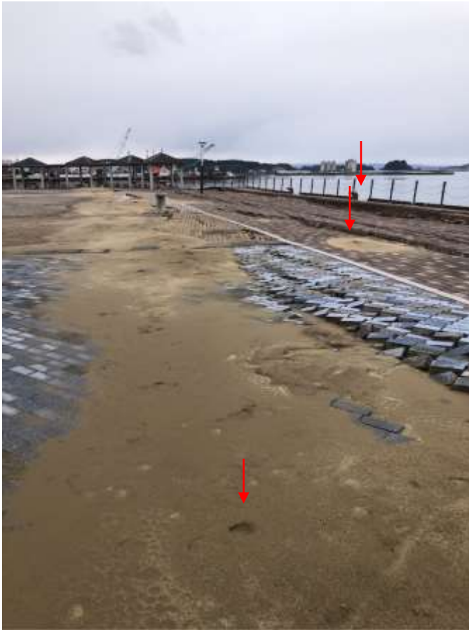
Tilted quay, sand ejecta and ground subsidence
