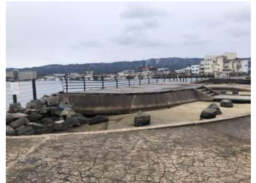
Subsidence and curved quay
