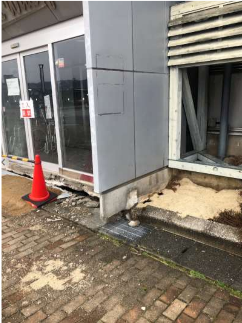
Ground subsidence and sand ejecta
