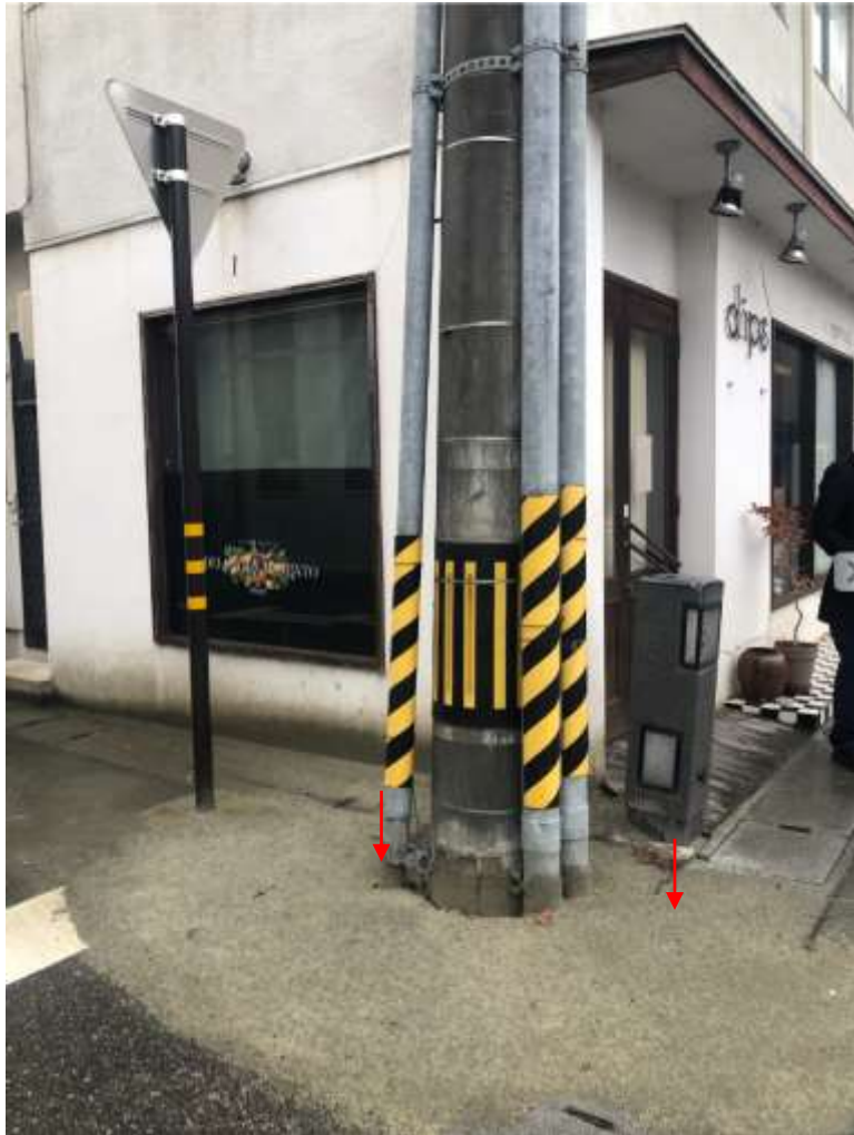
Pole settlement and sand ejecta
