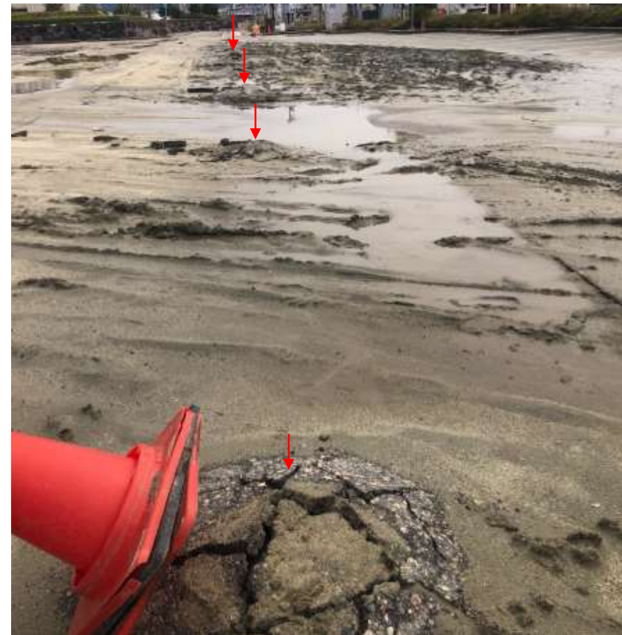
Manholes and pipeline uplift
