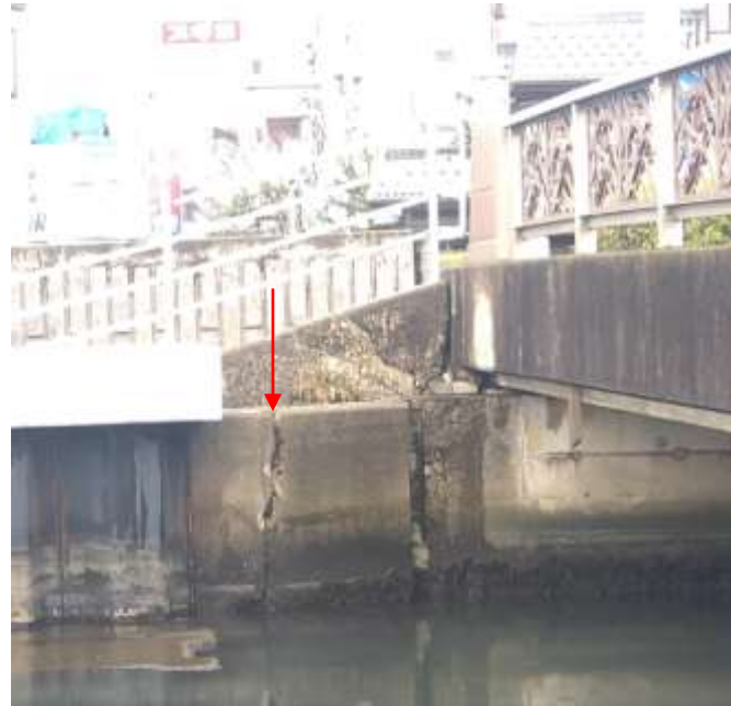
Cracks in bridge stairs
