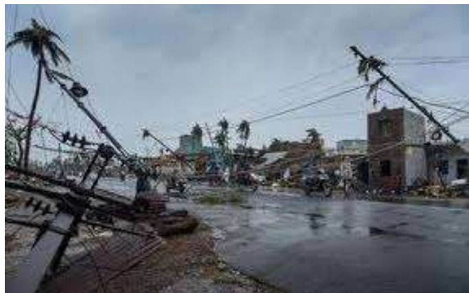
Aftermath of Cyclone, Devastation of electrical infrastructure Source: Outlook India, Date: 7 th May, 2019.
