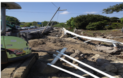
Photo 7: Ground failure along this road in Mashiki Town separated the guardrail from the roadbed
