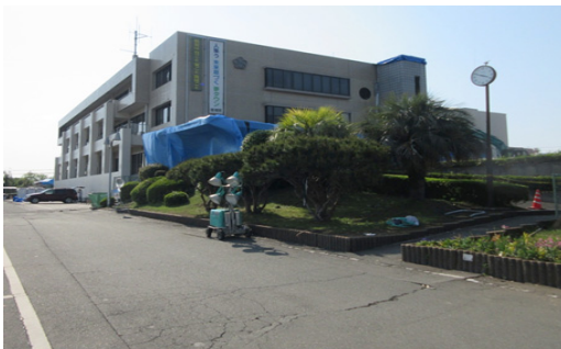
Photo 14: Mashiki Town administrative building (town hall) sustained structural and non-structural damage and was evacuated. April 29, 2016.
