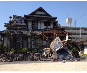
Photo 9 Partial collapse of older two-story house in southeastern area of Kumamoto City
