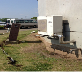
Photo 6: Ground failure and settlement around foundation
