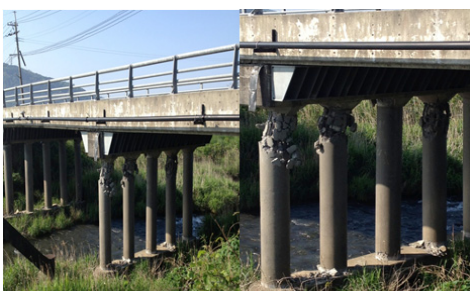
Photo 15: Column failure at highway bridge, Mashiki Town, May 1, 2016
