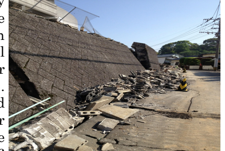
Photo 17: Another view of damaged and partially collapsed stairway and retaining wall Mashiki Town, May 1, 2016.
