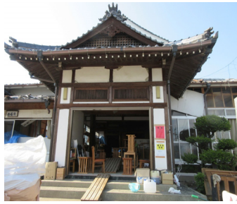
Photo 12: The Konkokyo Shinto Shrine in Mashiki Town is red tagged and portions of the building collapsed, April 29, 2016.
