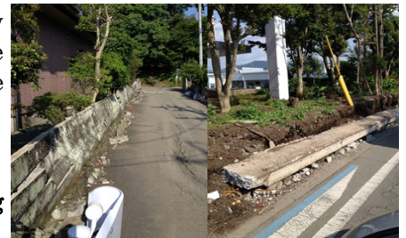
Photo 16: Damaged residential concrete walls, Mashiki May 1, 2016
