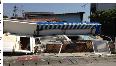
Photo 11: The complete collapse of this hair salon in southeastern Kumamoto City, April 30, 2016.
