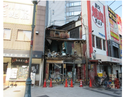
Figure 1: Damage to an old house in Osaka City.
